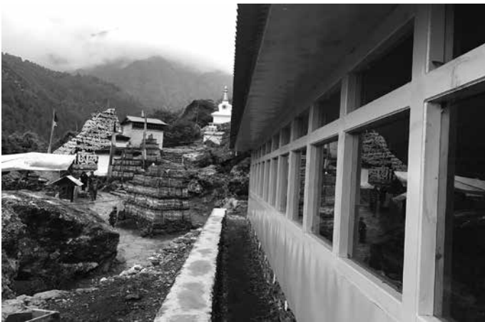
Students survey the site of the first public restroom in the Khumbu Valley, located in Ghat, Nepal. In the foreground is a school dormitory that Hike for Help built in spring 2017.
